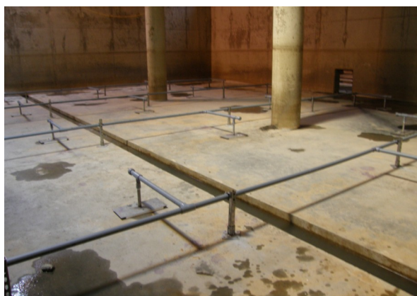
Bio M x tank installation at F. Wayne Hill WRC
